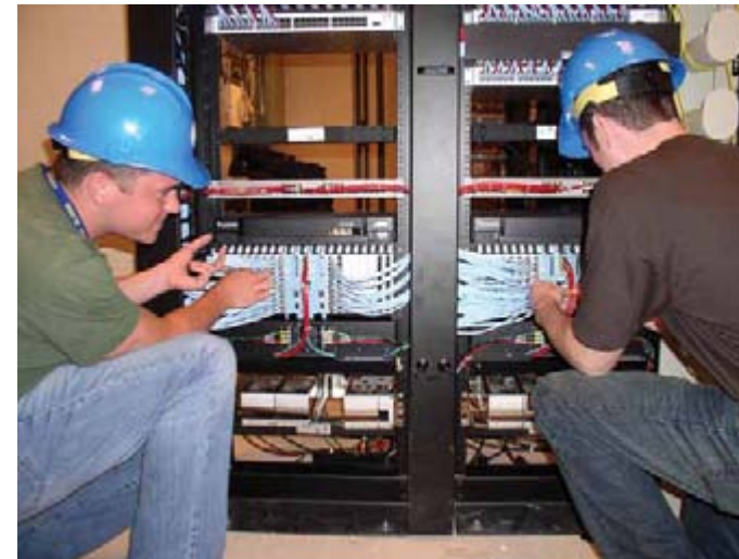
iMAP™ active fiber equipment installed at the MDF
